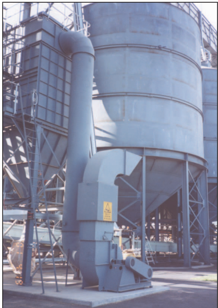
MAVA 320 fan, Arr.1, 45kw c/w discharge damper, silencer and elbow. Grain dust collection system.
